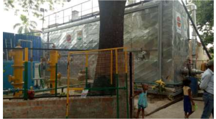
IDH Kjjakpura 5 TPD Plant
